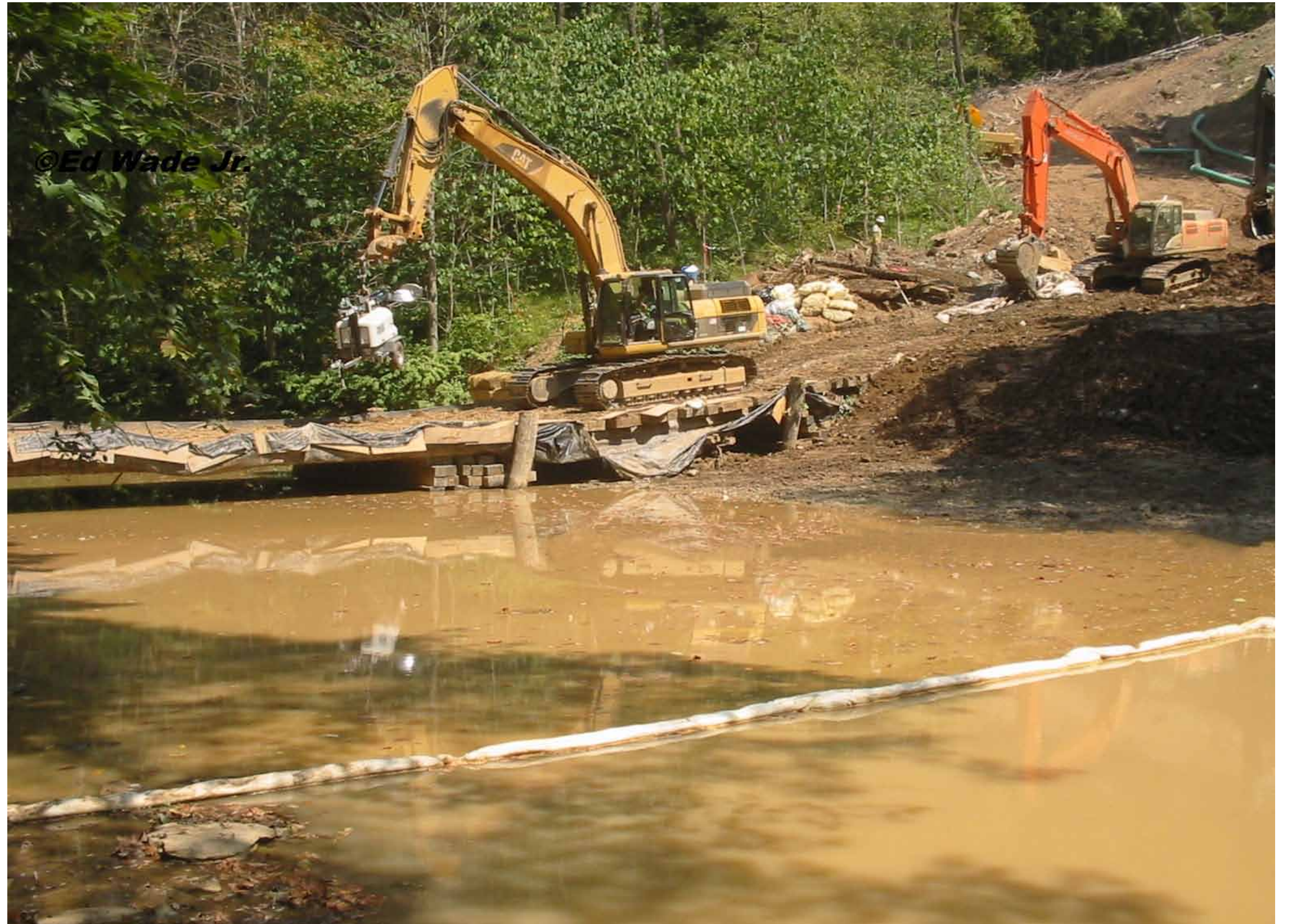
Pipeline construction crossing a stream in Wetzel County, WV. Photo by Ed Wade, Jr.
